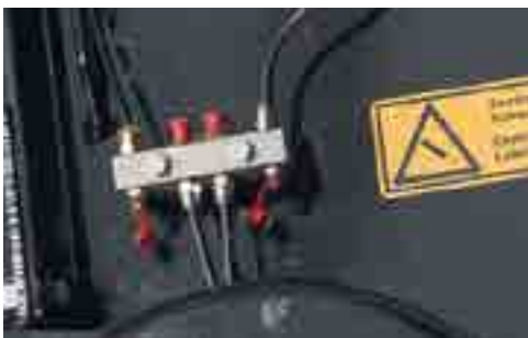
Central lubrication point
