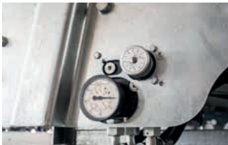
Mechanical feed control through mechanical potentiometer
