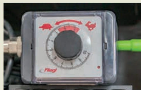
Electrical potentiometer with feed rate adjustment on control panel
